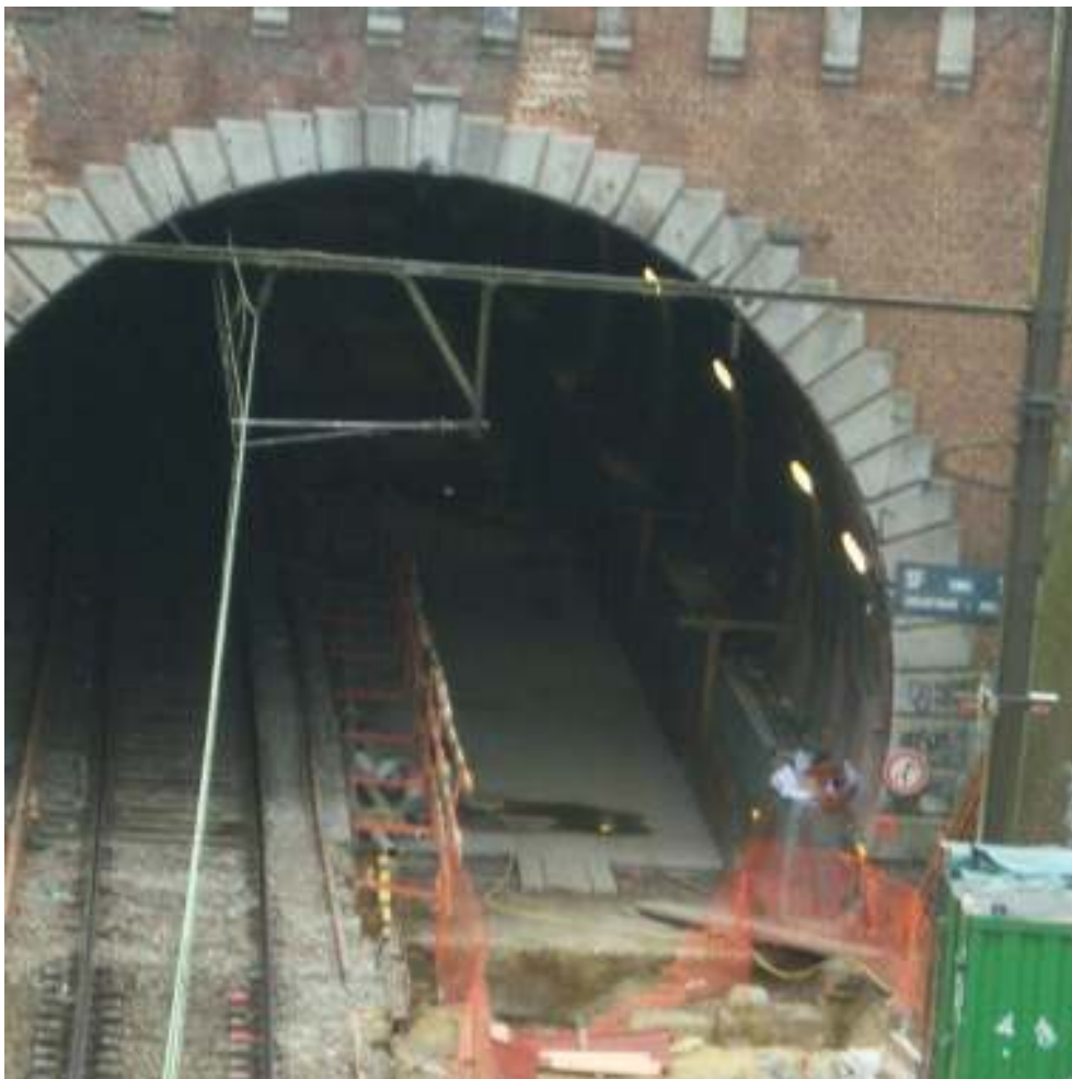
Work on the Josephat – Schuman tunnel, which will connect Brussels Airport to the European Quarter of the city and to Namur and Luxembourg
