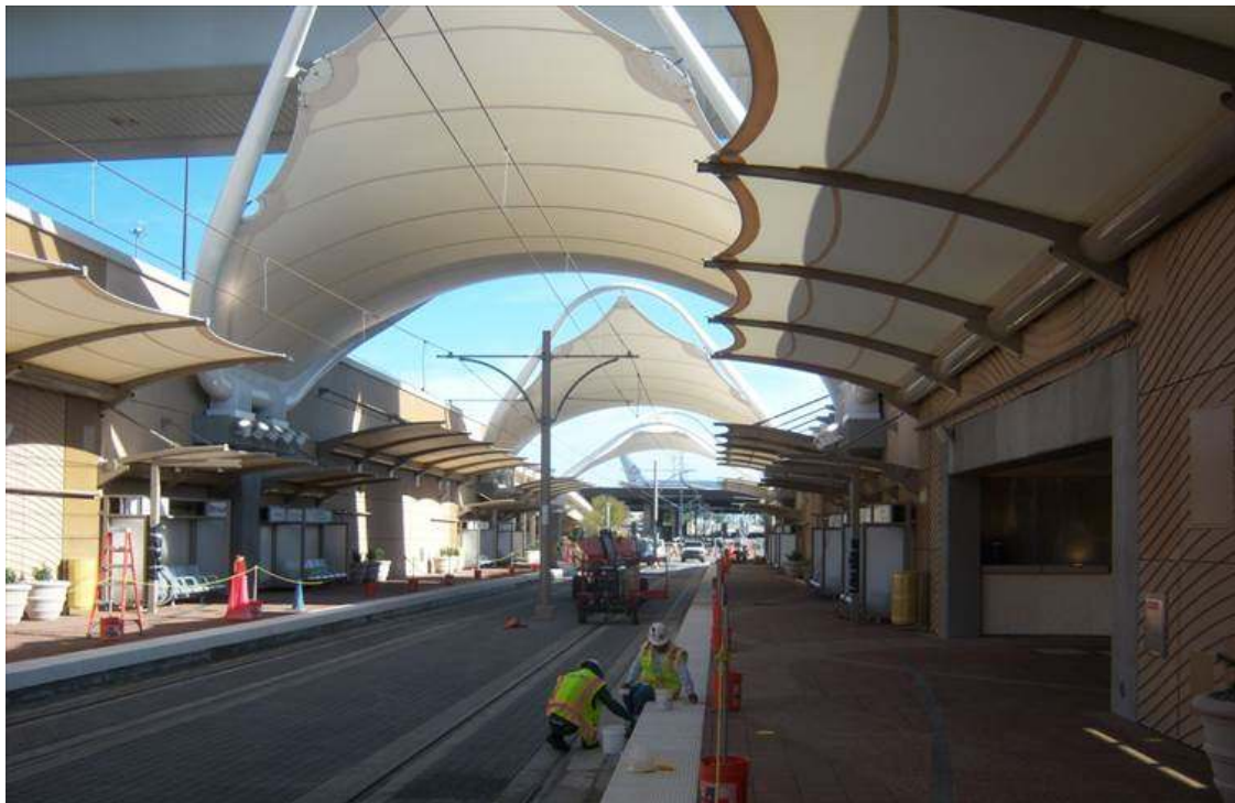
The new station on the DART Orange Line at Dallas Fort Worth Airport nearing completion at the time of the IARO workshop in April 2014
